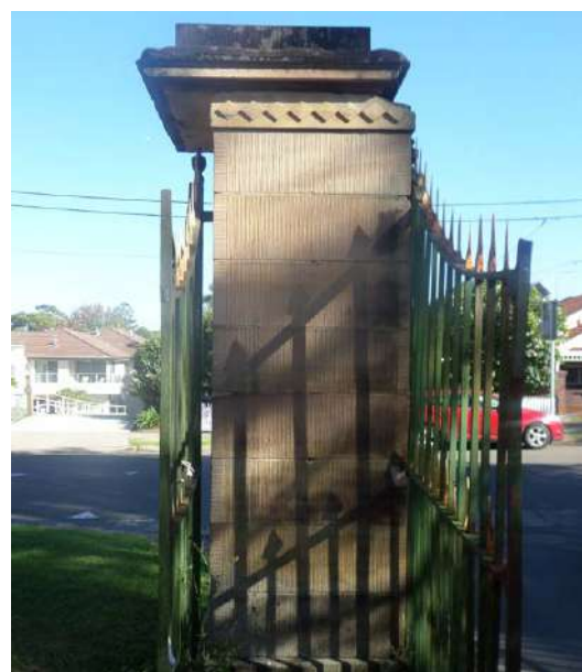
Top image: Punt Road Gateway following repairs Lower image: Punt Road Gateway stone pier prior to repairs
