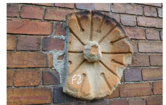
Top image: Façade following completion of repairs Lower image: Detail of damaged stone prior to repairs
