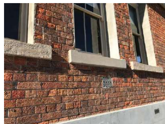
Top image: Bega PS during facade and chimney repairs Lower image: Replacement of damaged stone window sill
