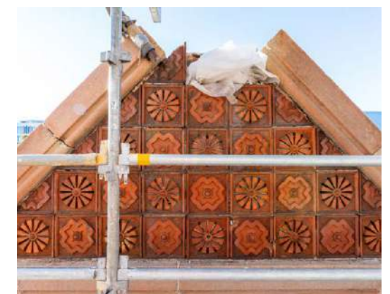
Top image: Completed Hunter Street facade Lower Image: Stone and terracotta tiled gable during repairs
