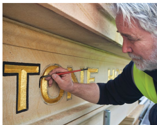
Top image: Completed conservation works to the Main entry of Denistone House at Ryde Hospital
