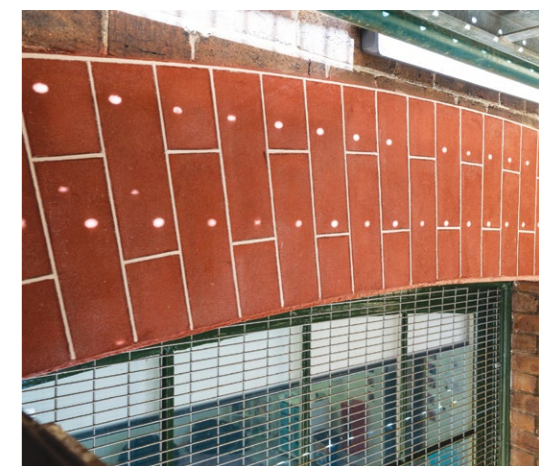
Top image: Decorative stonework to main entrance prior to the commencement of conservation works
