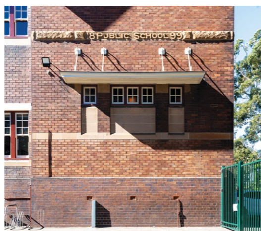
Top image: Gardeners Road Public School Lower image: Completed conservation works to window awning
