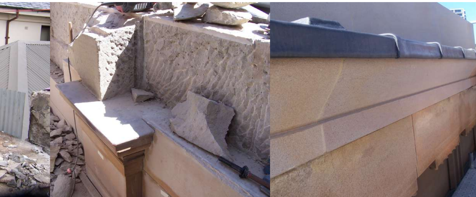
(left to right) Removal of the coping, cutting out the existing deteriorated cornice, completion of the project, Darlinghurst Court.
