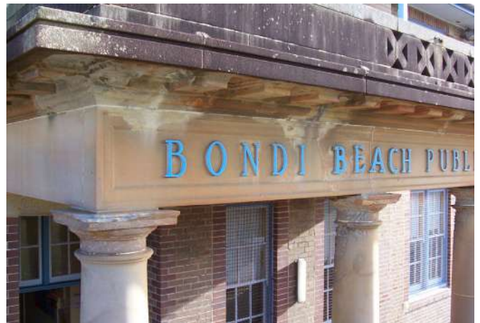
Deterioration of stone elements of the entrance portico at Bondi Beach Public School.
