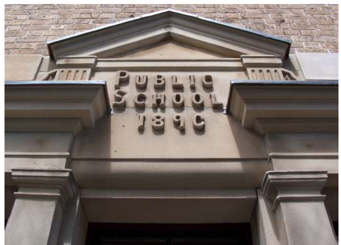
New stone repairs and lead weatherings to south west elevation (chapel street), Marrickville Public School.
