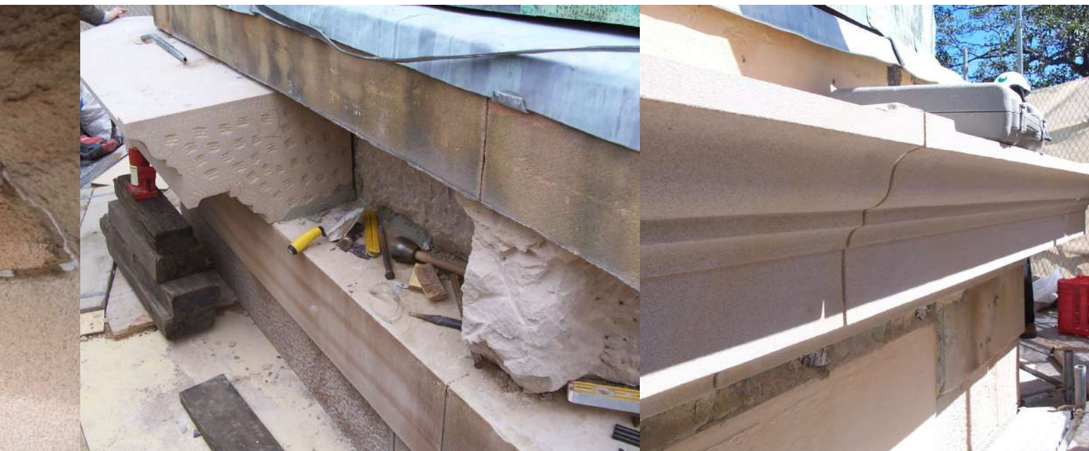
(left to right) Severely deteriorate cornice stones, new processed cornice stones being fixed, all cornice stones fixed awaiting pointing, Sydney Observatory.
