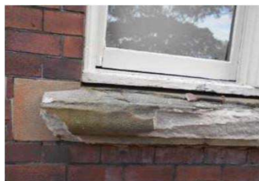
Top image: Heritage Architect Anita Krivickas and Site Controller Jordan West inspect the work to the windows Lower Image: deteriorated high level stone window sill
