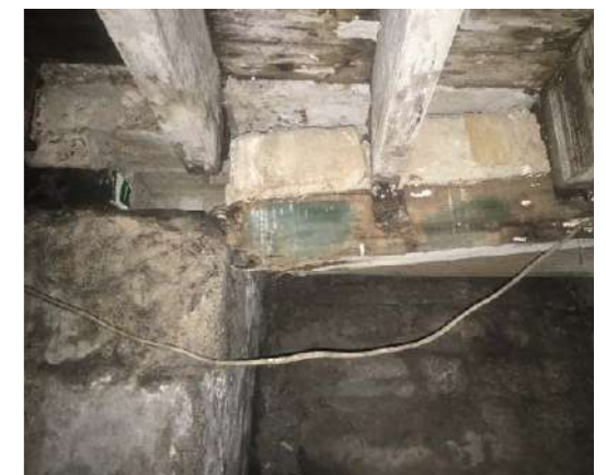
Top image: View from basement of original Level 1 floor joists, ends have been spliced with new timber notched into replacement timber window lintels and wall plates holding up the external stone walls. Lower Image: Rotten and collapsed timber substructure for external stone walls
