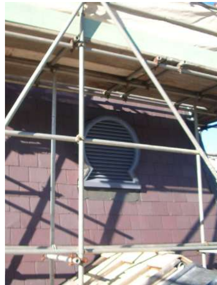
Reconstruction of the slate roof and timber roof vents at Royal Prince Alfred Hospital
