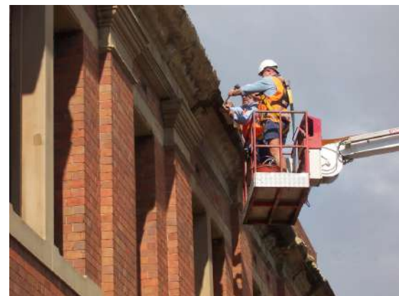
Stone Safety Inspection of the cornice of the Office Building at the Powerhouse Museum
