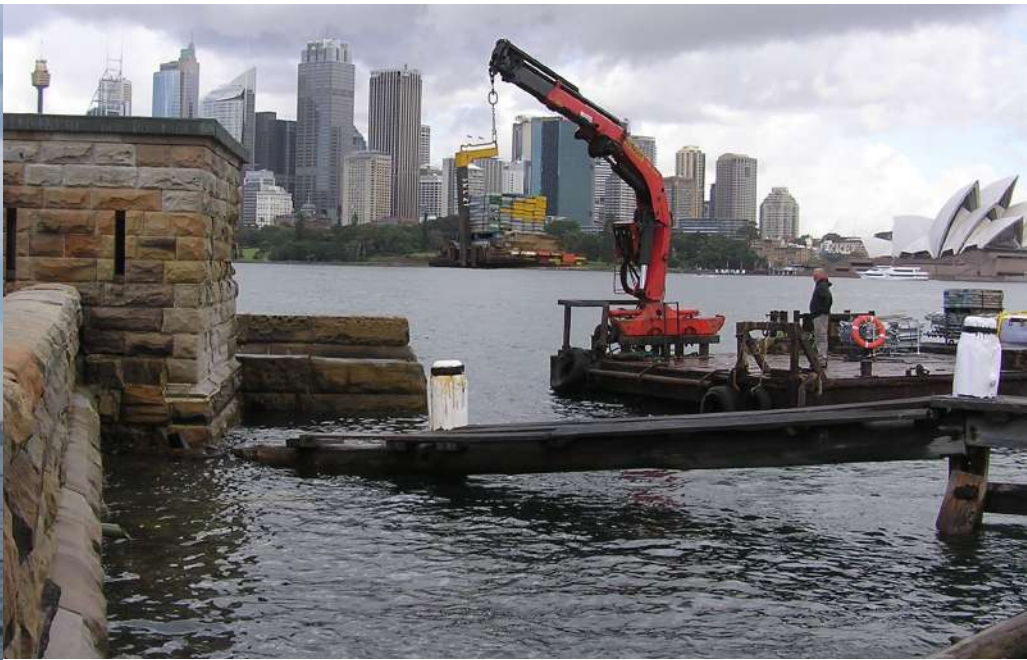
(left to right) Fort Denison on approach, delivery of stone and construction materials by barge for conservation works to the Slipway, Fort Denison, April 2008.
