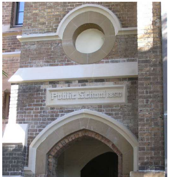
Paddington Public School Oxford Street Entry, 1856 date stone was recarved and fixed in 2007
