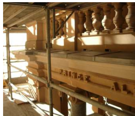
Replacement of the projecting cornices and installation of protective lead weatherings at Royal Prince Alfred Hospital
