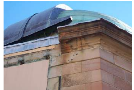
Sydney Observatory north dome deteriorated cornice
