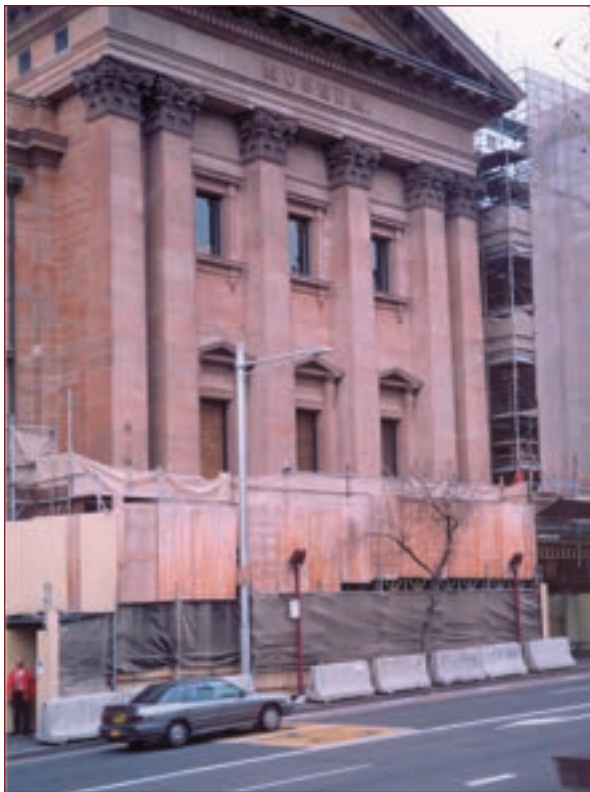
Birdproofing not visible from street
