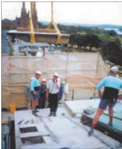
Above: Lowering a section of the pediment into place. The steel straps hold the pediment together.
