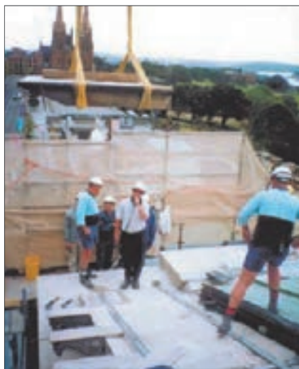
Above: Lowering a section of the pediment into place. The steel straps hold the pediment together.
