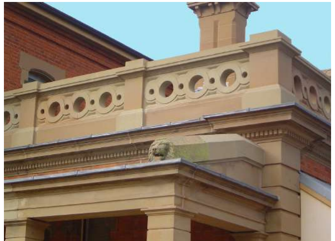
Completed stoneworks to western portico on Elizabeth Street including replaced Gullioche patterned balustrades.
