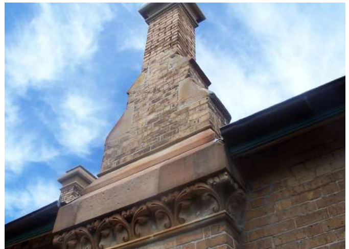
Paddington Public School - Work Area 4 Chimney flue buttress delaminated and requiring replacing. Chimney flu plinth stone to be indented.
