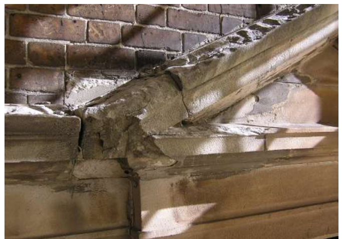
Marrickville Public School - pediment above main entry severely deteriorated.
