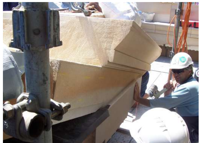
The springer stone is complex to remove, process and subsequently fix back into position. It requires the knowledge of skilled stonemasons to perform this challenging task.
