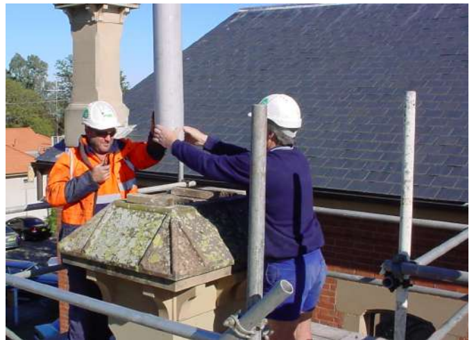
Stabilisation works to chimney. Stainless steel tubes are attached to sound structure below the chimneys and concrete grout placed around the tube.
